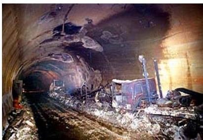
Mont Blanc Tunnel fire on March 29, 1999
